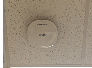
(a) Aruba AP-635 access point serving the campus network.
