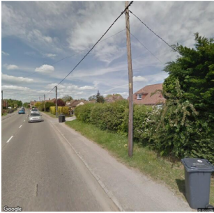
(a) Wooden utility pole
