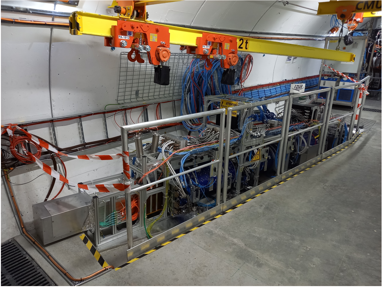
Figure 3.9: The FASER detector after installation in TI12. (This figure is taken from Ref. [34].)
