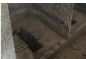
Scene: bathroom V/A/D: 1 / 8 / 5 Caption: A severely neglected and filthy public bathroom with heavy grime, stained concrete, and highly unsanitary conditions, triggering an immediate and intense visceral reaction of sanitary disgust.
