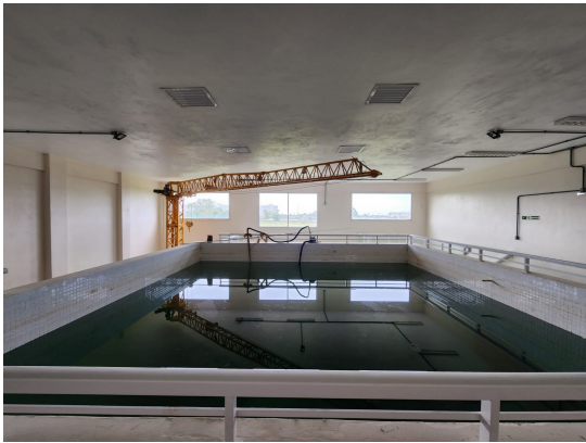
Fig. 2: Indoor Tank Facilities.
