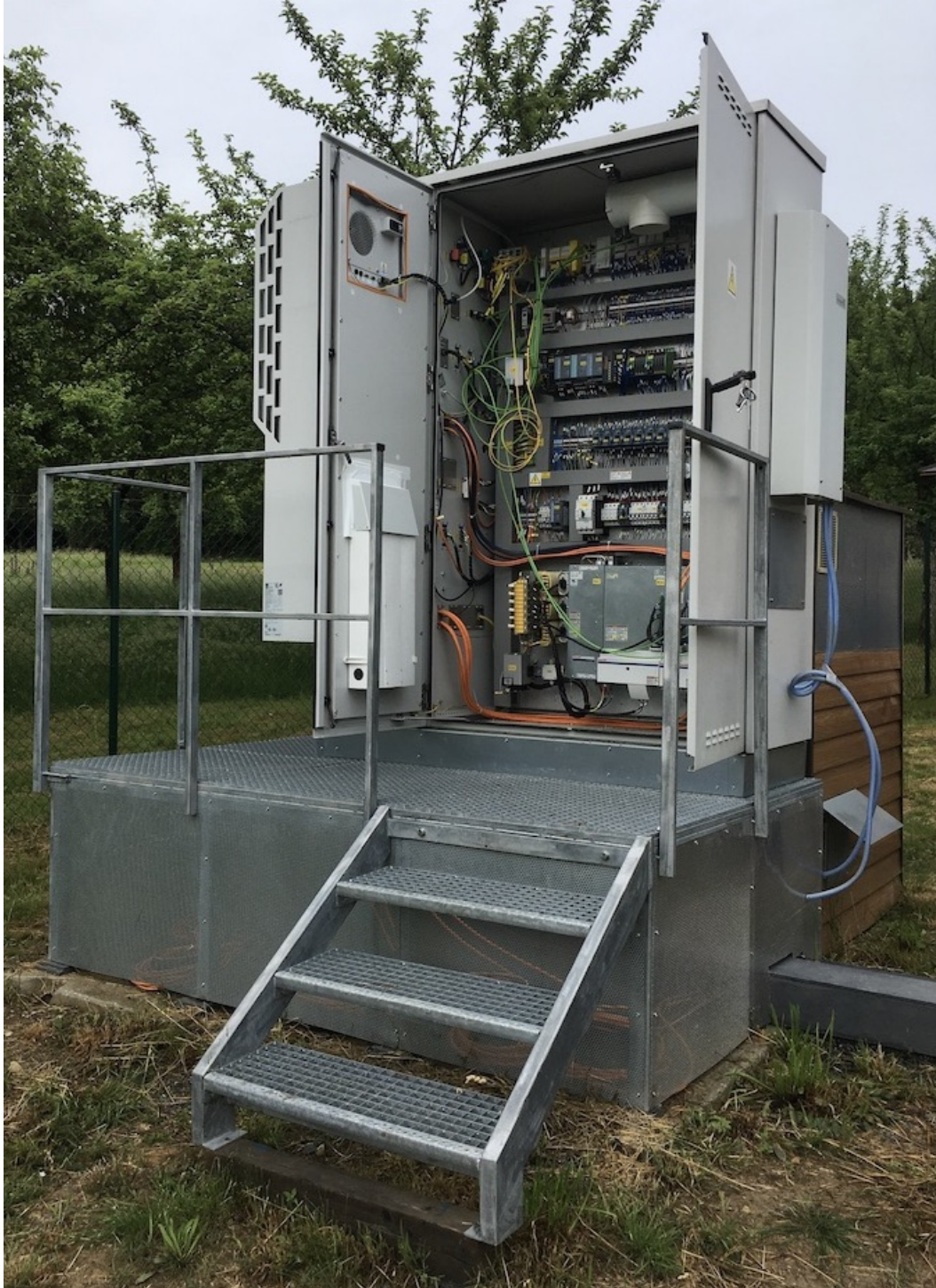
Figure 40. Control cabinet of the prototype telescope.
